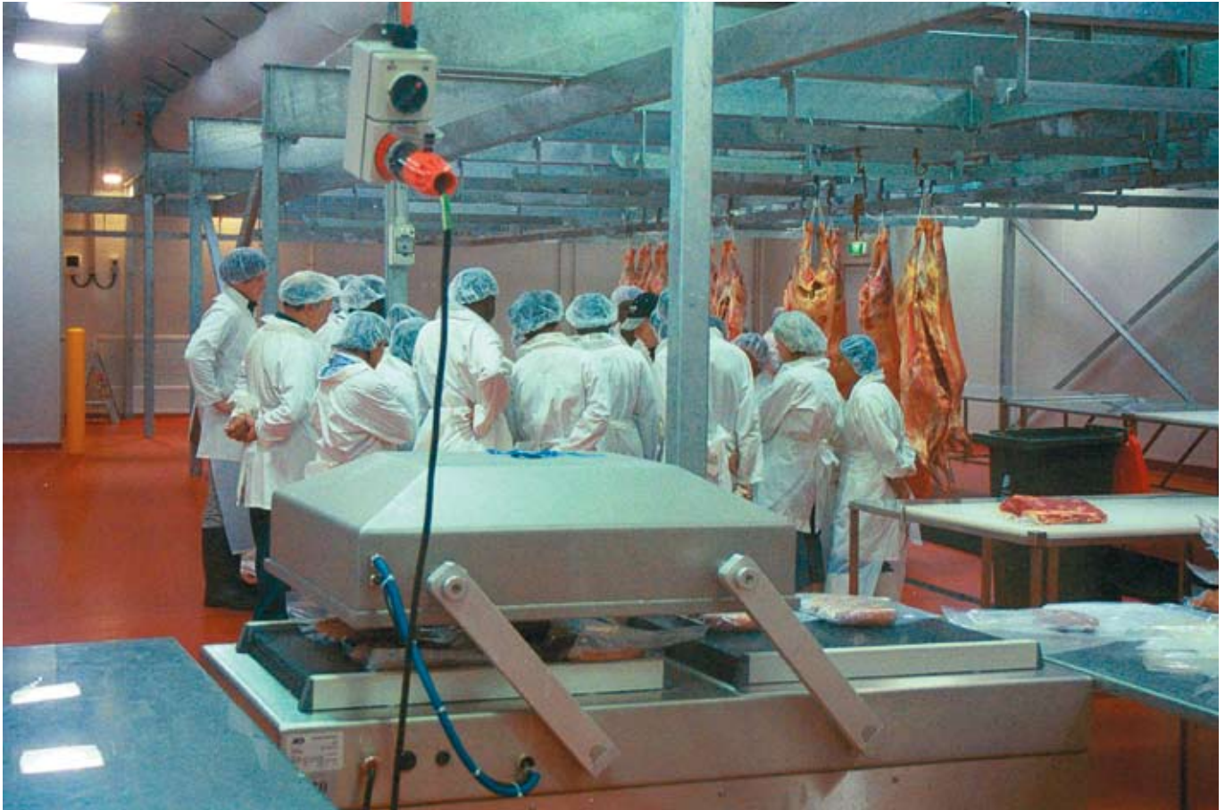
The NMIT meat processing facility has chillers, freezers, 16 boning stations as well as sausage making equipment and vacuum packers.
